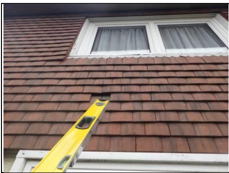
Missing tile to front
