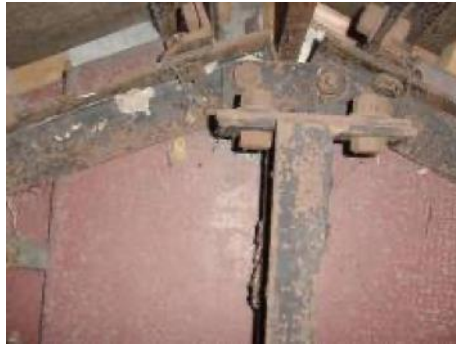
Rusting to a lightweight metal frame or damage or deterioration to the metal frame of a non-traditional house
