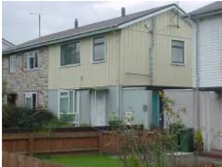
BISF property with metal profile sheet roof (has asbestos roof been removed or has it been overclad?) and metal profile sheet at first floor level and render at ground floor level and older style double glazed windows
