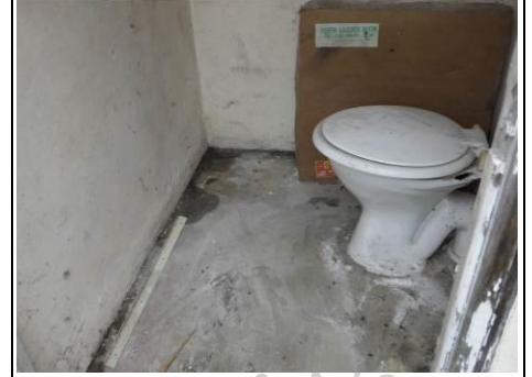
Dampness around toilet
