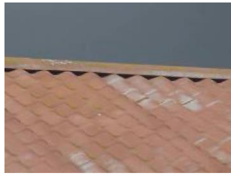
Weathering effect to roof
