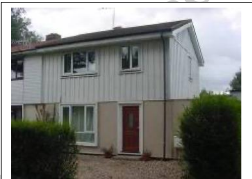
Metal frame house with profile metal sheeting at top and render at bottom. Roof has been changed.
