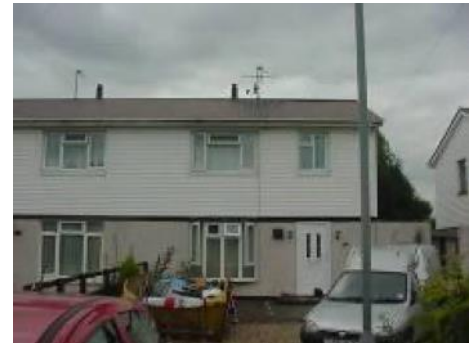
BISF house with a profile metal roof, (again has asbestos roof been removed?), plastic cladding at first floor level (is there insulation between the profile metal sheets and the plastic cladding that is causing condensation) with pebbledash render at ground floor level and modern double glazed windows
