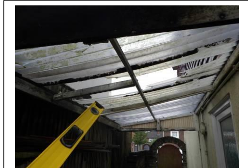
Deteriorating corrugated plastic roof to right side
