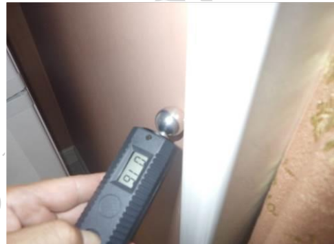
Unable to obtain lateral damp readings due to dry lining
