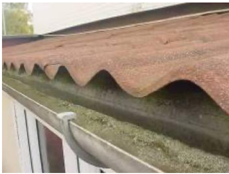
Close up of edge of profile metal roofing that looks like a tile
