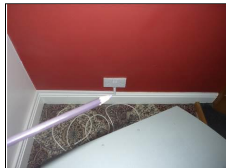
Some surface wiring should be boxed in
