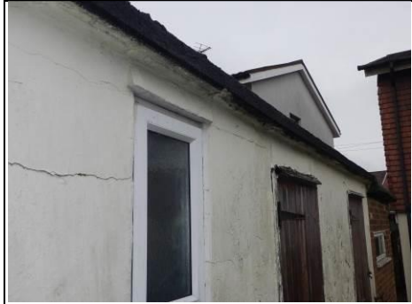
Cracking to outbuilding walls
