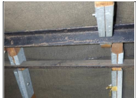
Rusting to some of the angle irons
