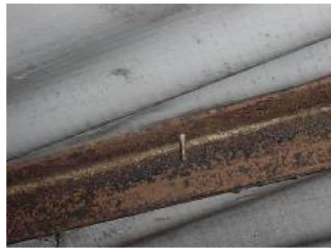
Example of rusting that we have seen in the roof of a metal framed building
