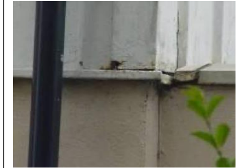
Rusting to profile metal cladding
