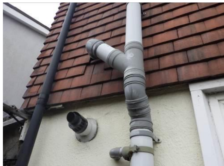
Soil and vent pipe close to flue
