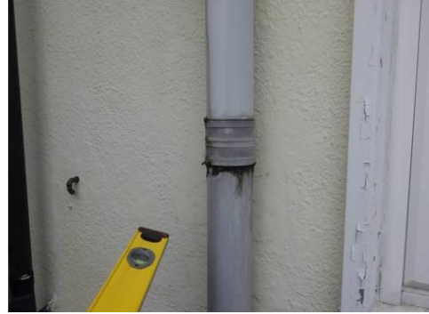
Soil and vent pipe leaking slightly
