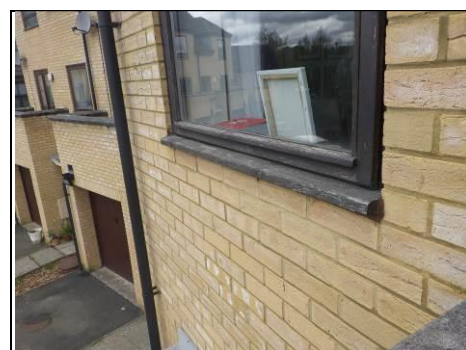
Flaking paint and bare timber
