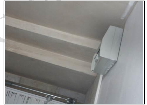
Fuse board in garage
