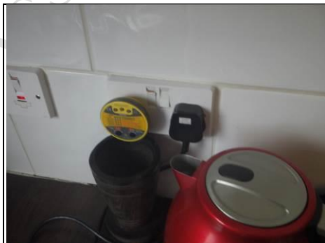
Earth test failed
