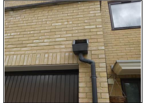
Hopperhead to balcony
