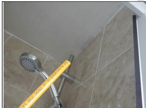
Black mould painted over and deteriorating paintwork
