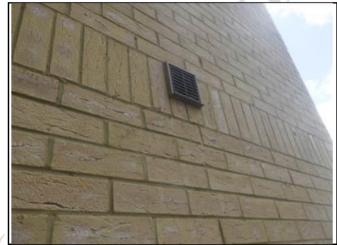
Extract vent from WC
