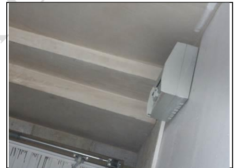
Fuse board in garage
