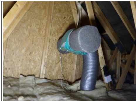
Left gable plywood with positive pressure extract fan
