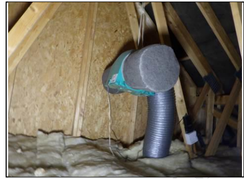
Positive pressure fan in roof space
