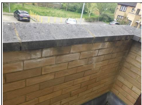
Balcony wall damp
