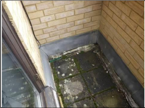
Dampness to balcony
