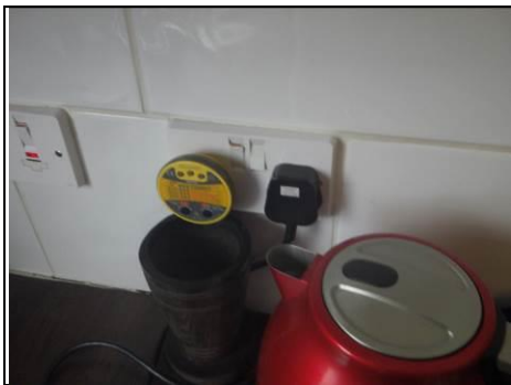
Earth test failed
