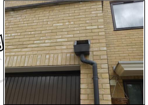
Hopperhead to balcony
