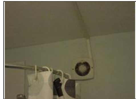
Small extract fan needs to be improved
