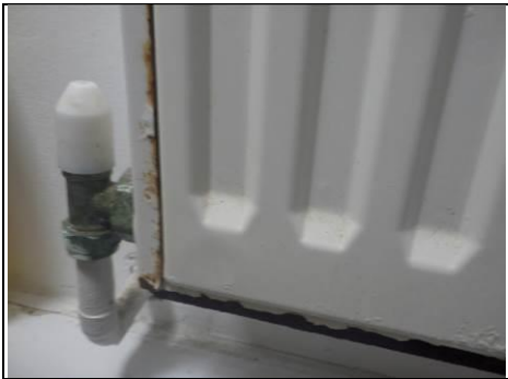
Radiator rusting due to dampness
