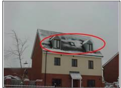
Heat loss via poorly insulated roof
