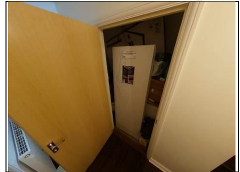
WC left full of stored items
