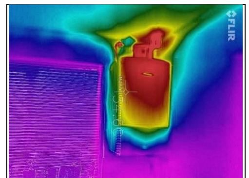
Boiler (Not your property)
