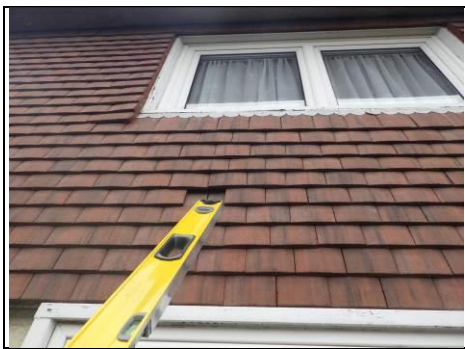
Missing tile to front
