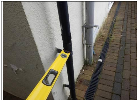
Running gully to rear
