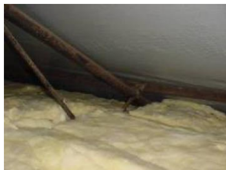
Example of over insulation of a metal framed property which causes condensation
