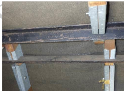
Rusting to some of the rolled steel angle
