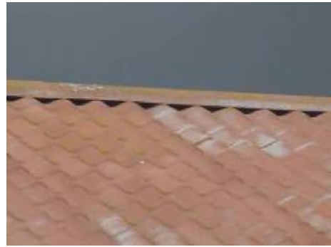
Weathering effect to roof
