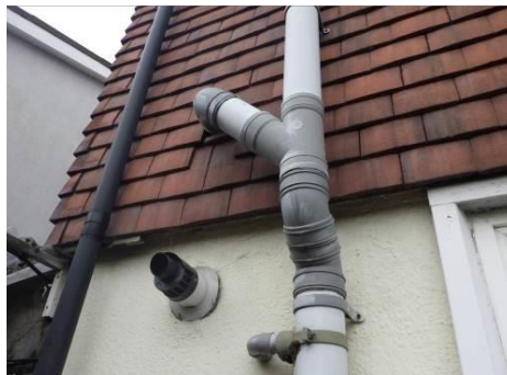
Soil and vent pipe close to flue
