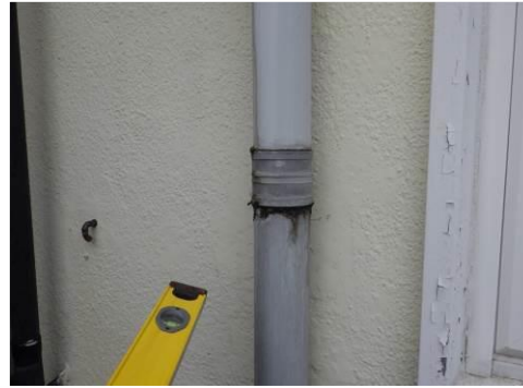
Soil and vent pipe leaking slightly
