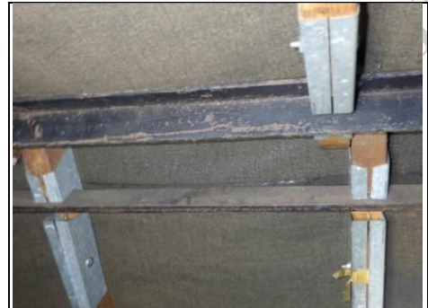
Rusting to some of the angle irons
