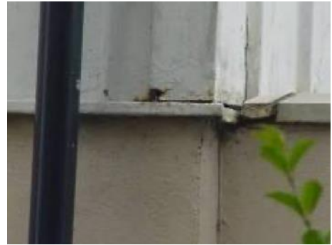
Rusting to profile metal cladding
