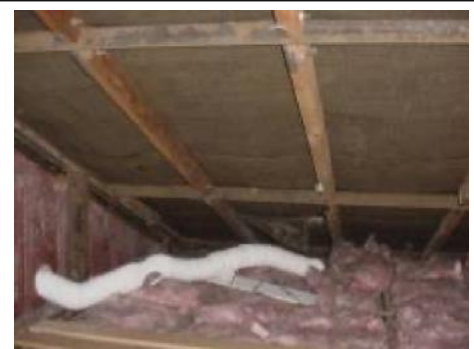
Extract vent to outside often discharges into roof which is essential that they do not in this type of roof
