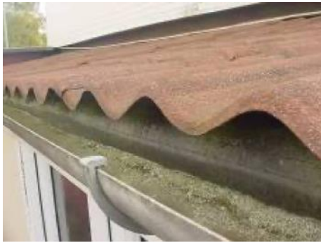
Close up of edge of profile metal roofing that looks like a tile
