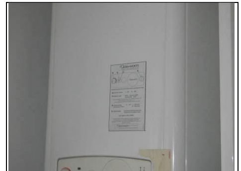
Glow worm boiler
