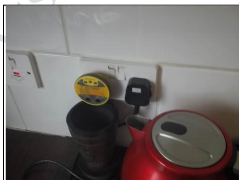
Earth test failed
