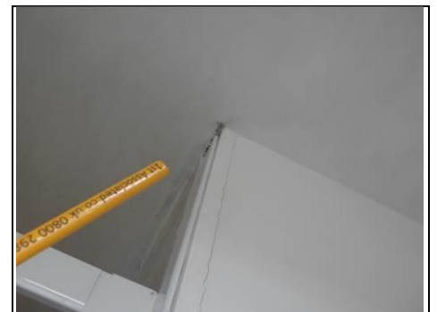
Black mould and hairline crack in plaster of en-suite
