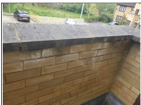
Balcony wall damp
