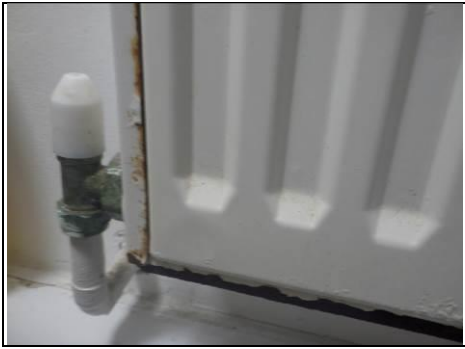
Radiator rusting due to dampness
