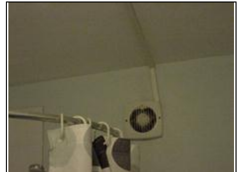
Small extract fan needs to be improved
