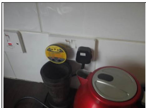
Earth test failed
