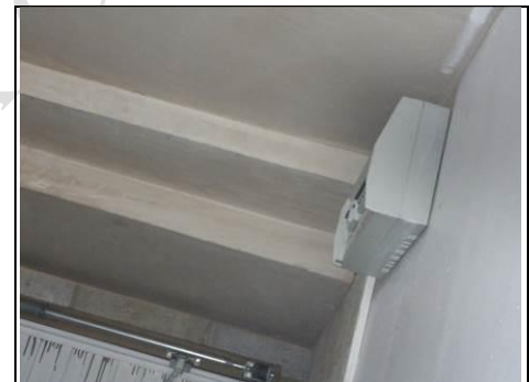
Fuse board in garage
