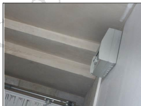
Fuse board in garage
