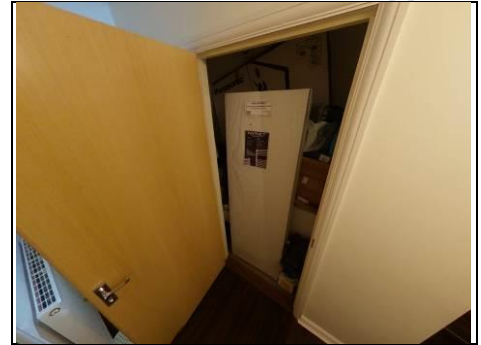
WC left full of stored items
