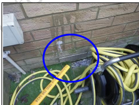
Rear airbrick acting as gutter
