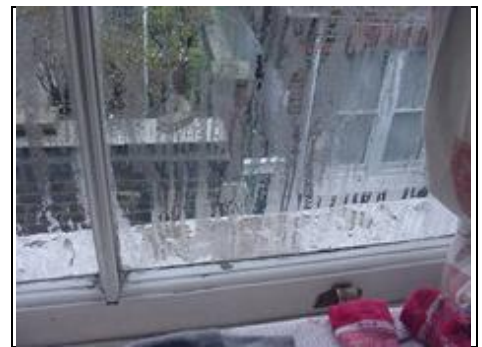
Condensation on window
