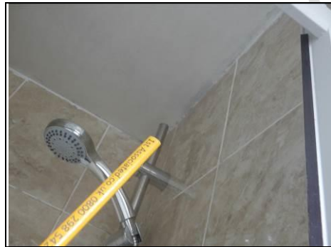
Black mould painted over and deteriorating paintwork
