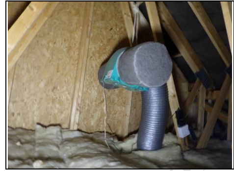
Positive pressure fan in roof space
