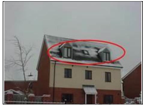
Heat loss via poorly insulated roof
