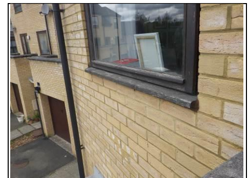
Flaking paint and bare timber
