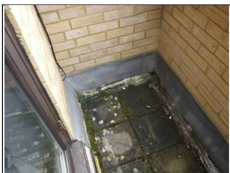
Dampness to balcony
