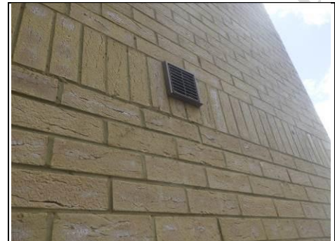
Extract vent from WC
