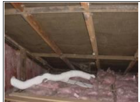
Extract vent to outside often discharges into roof which is essential that they do not in this type of roof
