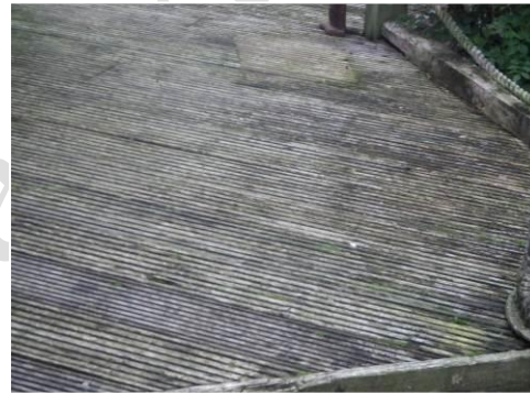
Moss on decking
