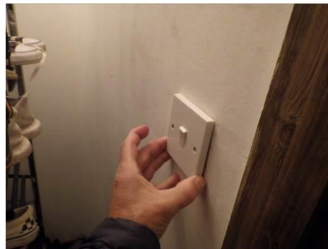
Light socket loose
