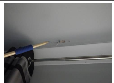
Dampness or condensation in main bedroom
