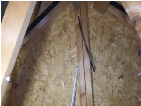
Example of timber frame structure visible in the roof space (Not your property)
