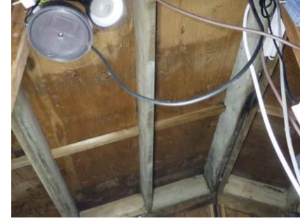
Dampness to main roof
