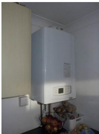
Glow worm boiler in utility room
