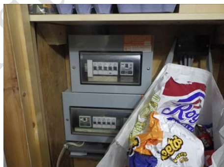
1980's-2000 fuse board in kitchen
