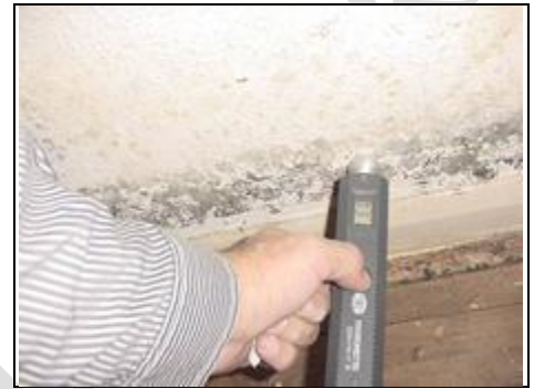
Black mould and high damp meter readings
