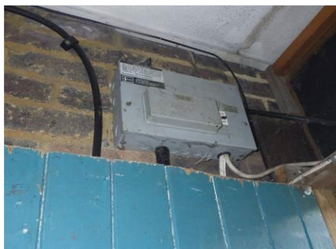
1960's-1980's Fuse board in right side area
