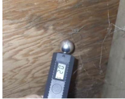
High damp meter reading of 120 in roof
