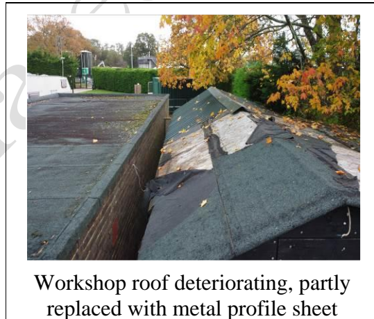
Workshop rotting sterling board in roof needs redoing
