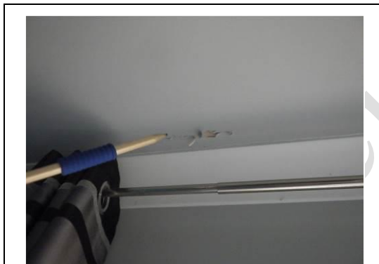
Dampness or condensation to main bedroom on rear left
