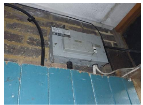
1960's-1980's Fuse board in right side area
