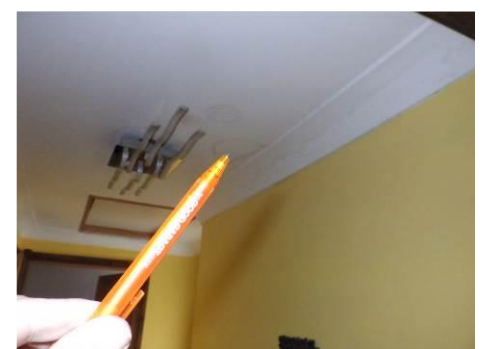
Water leak from toilet
