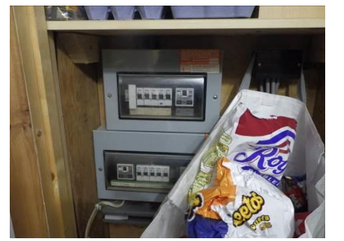
1980's-2000 fuse board in kitchen
