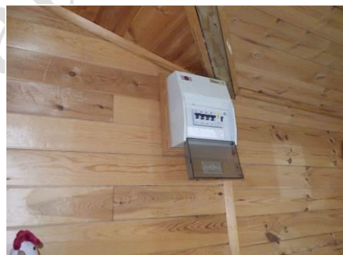
Electrics in bar
