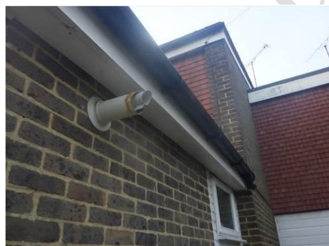
Flue from boiler
