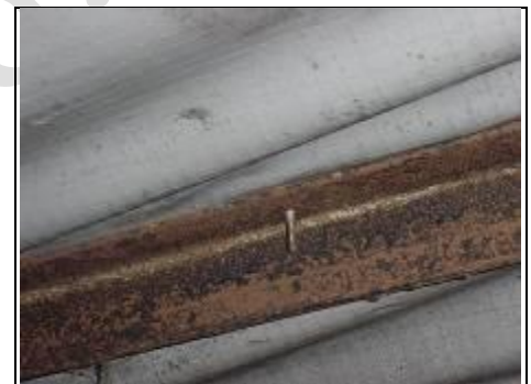
Rusting within the roof between the insulation and plastic protective underlayer
