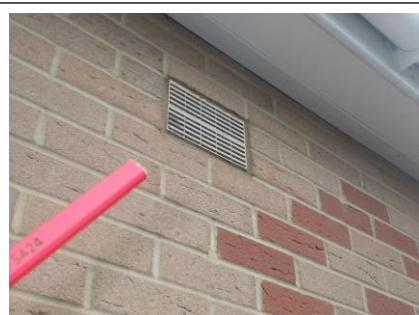
Air vent from kitchen on left hand wall
