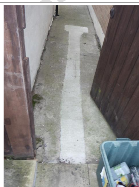
Area dug up due to electric problems
