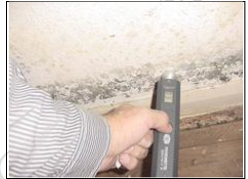
Black mould and high damp meter readings
