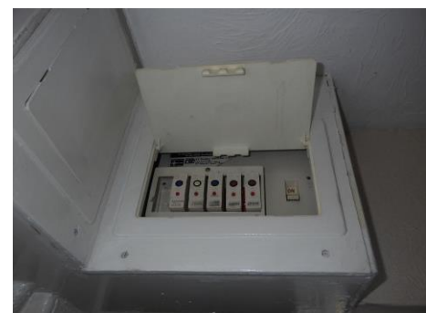
1980's-2000 fuse board
