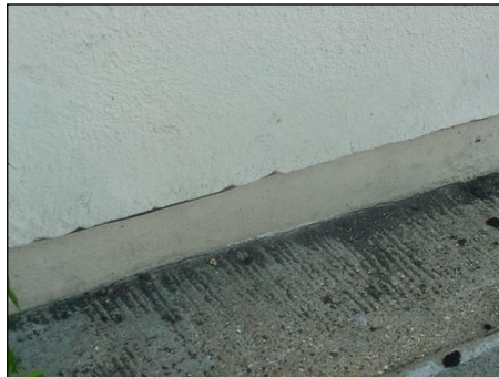
Drains repaired within passageway -looked to be on neighbours side
