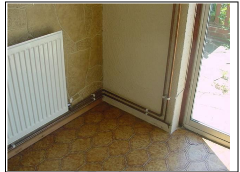
Surface mounted pipes
