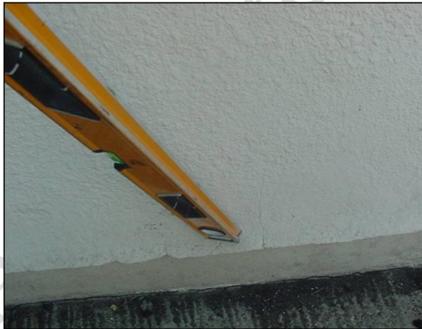
Vertical cracks indicating possible subsidence
