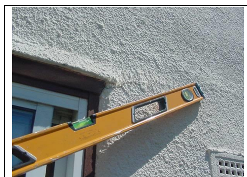
Crack to the rear sliding door
