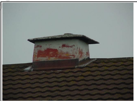
Asbestos original chimney non traditional house
