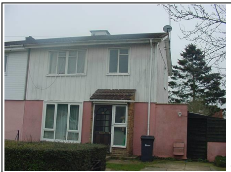
Painted cladding to non-traditional property
