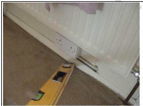
Surface mounted electrics
