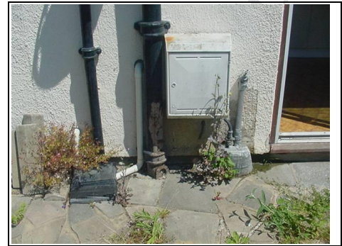
Gas cupboard to rear of property
