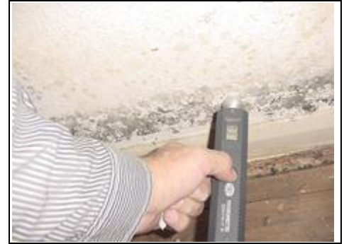
Black mould and high damp meter readings
