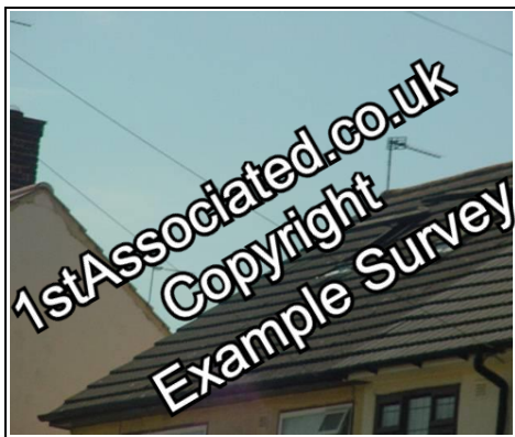
Roof windows to neighbouring properties
