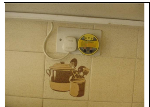
Electricity turned off
