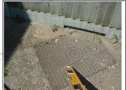
Manhole double sealed to front of property that we could not unscrew
