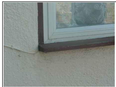
Front windows are older style plastic into timber with no trickle vents
