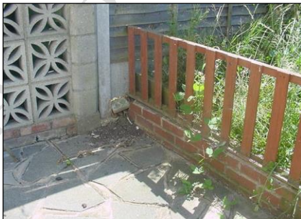
The boundary wall doesn't have any weep holes
