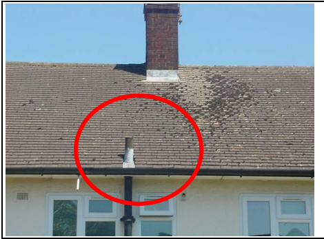
Soil and vent pipe
