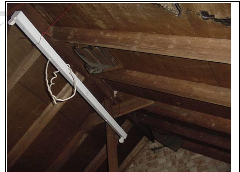
Light not working
