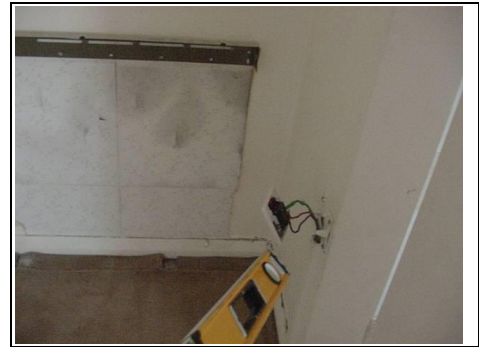
Electrics off wall in front bedroom
