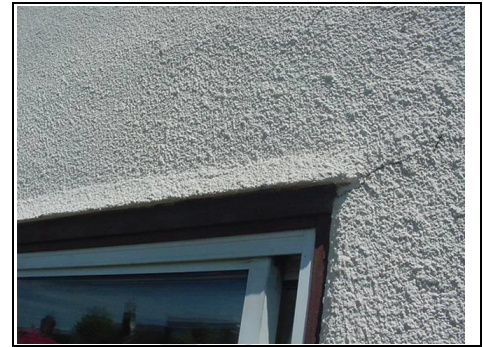
Drip over the window to the rear sliding doors
